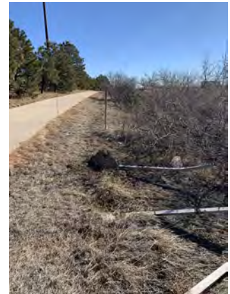
Image: Damaged Fence
