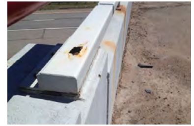
Image: Rusted Metal On Bridge Rail
