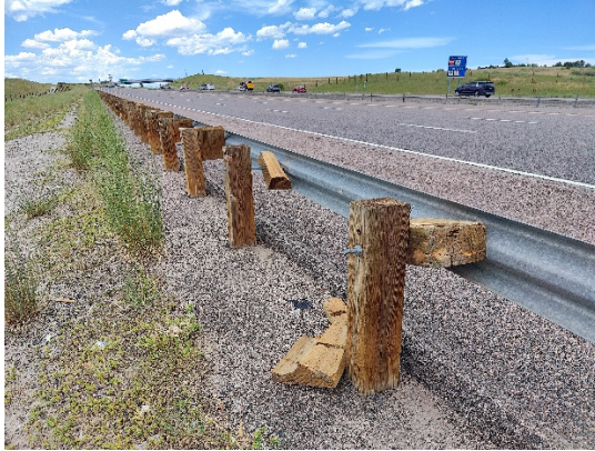
Figure 2-9 – Broken wooden posts (typ.)
