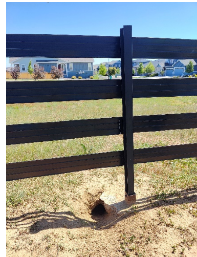
Figure 2-17 – Another Prairie Dog tunnel at snow fence post foundation
