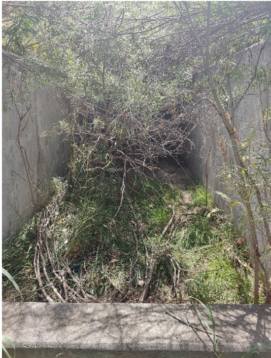
Figure 2-6 – CBC at MP 7.25 with significant foliage and overgrowth at the inlet
