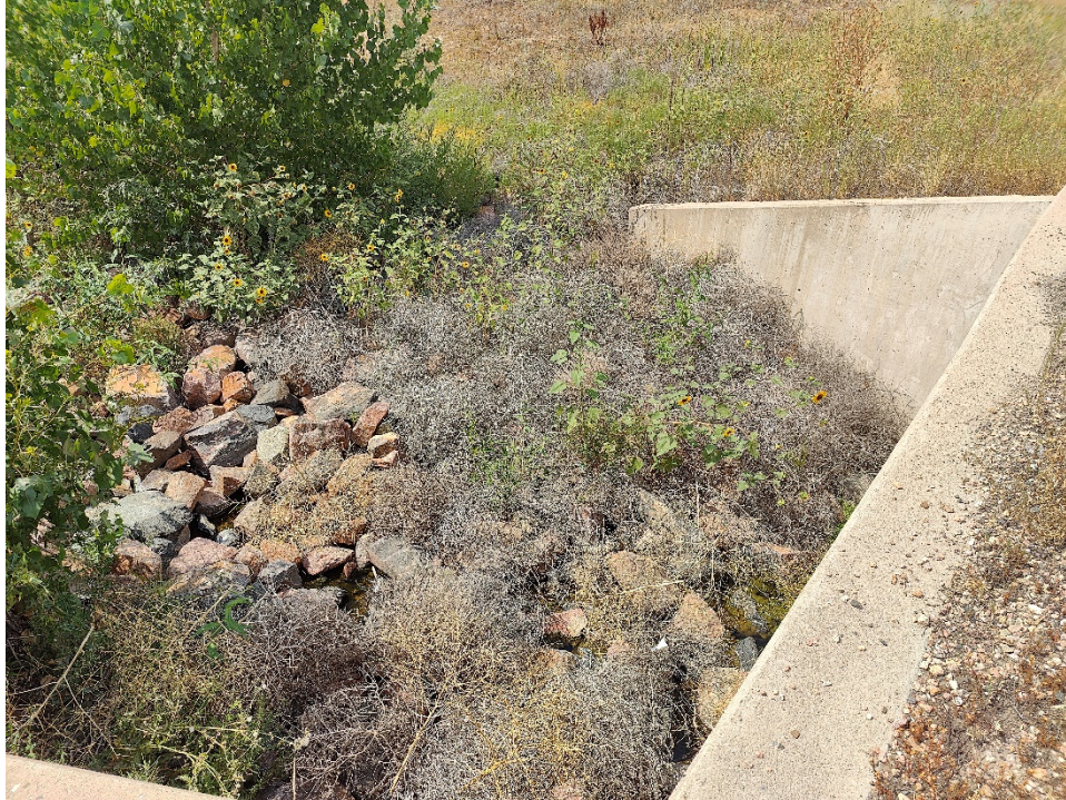
Figure 2-5 – Start of tumbleweed collection at outlet of CBC north of Tower Road
