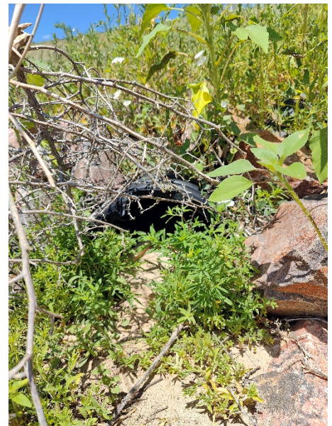
Figure 2-19 – Heavily blocked and overgrown EP outlet at 104 Ave.
