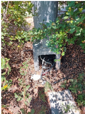
Figure 2-1 – Open access panel with wires exposed, SB Chambers Off Ramp
