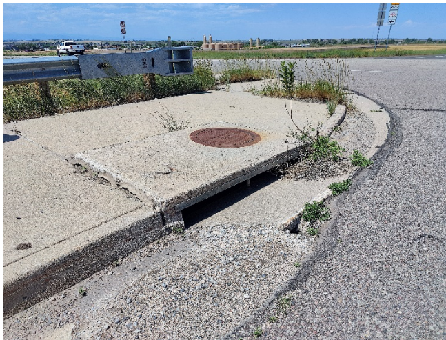
Figure 2-18 – Settling and concrete warping at EP inlet at Colorado Blvd. Exit
