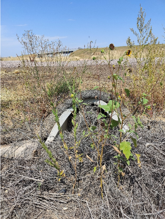
Figure 2-7 – Culvert south of SH 30 with significant tumbleweed blockage at inlet
