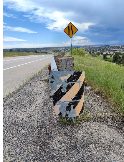
Figure 2-10 – Scraped and fading marker paint on guardrail along SB Smoky Hill On Ramp
