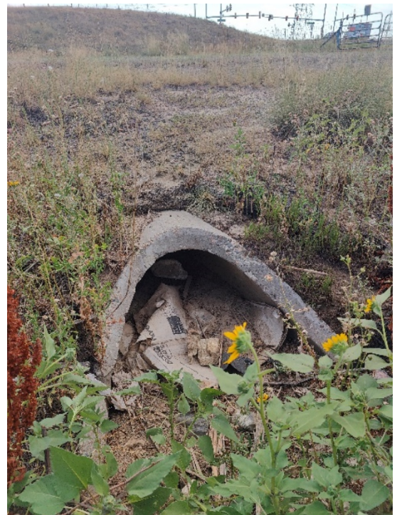
Figure 2-4 – Outlet of the culvert in Figure 2-3, displaying sediment and trash blockage
