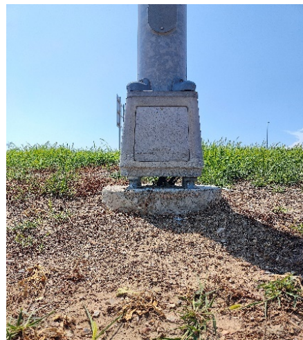
Figure 2-2 – Pole with observed gap between foundation and base
