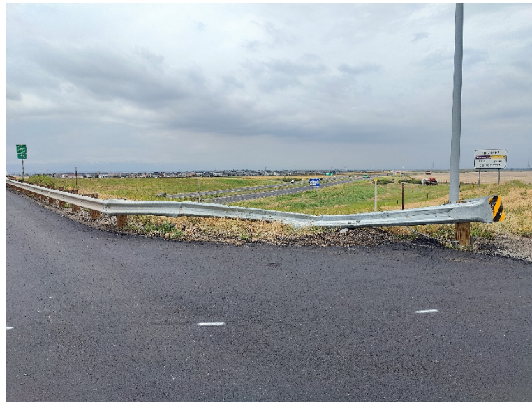
Figure 2-8 – Collision damage to guardrail at 96 th Ave NB ramp
